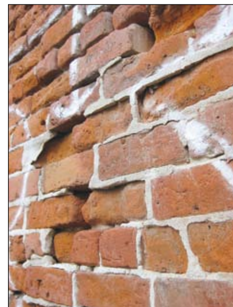
Portland cement mortar results in eroded and structurally unsound brick. These bricks have lost their strong outer face in a process known as spalling.
