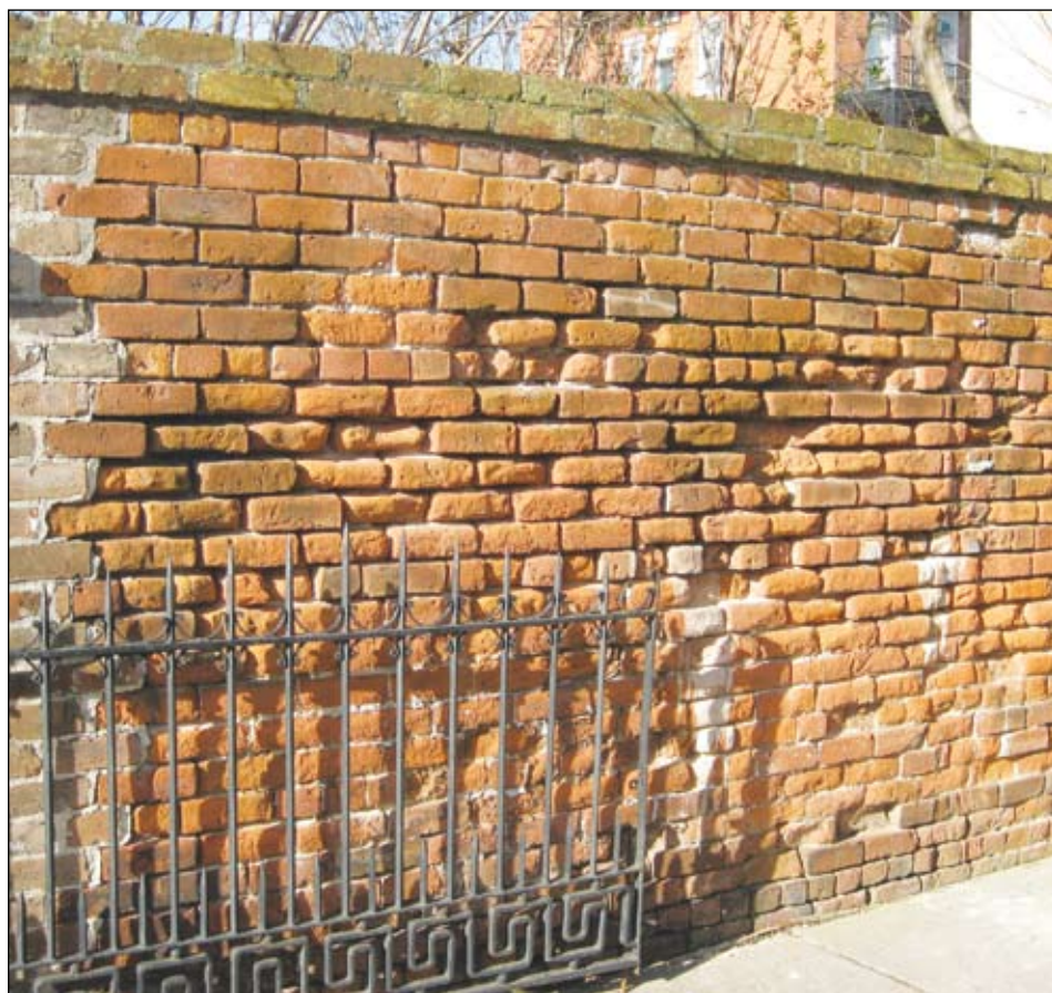
Improper maintenance, or a lack of maintenance, results in brick mayhem.
